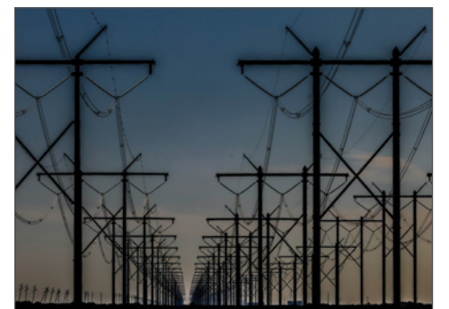
An SFI working group met in February to discuss the various coinciding pressures on the U.S. electrical grid and the changes to governance that might be needed to address those challenges. (image: Overhead power lines crossing the Everglades. Greg Stellentin/Unsplash)
